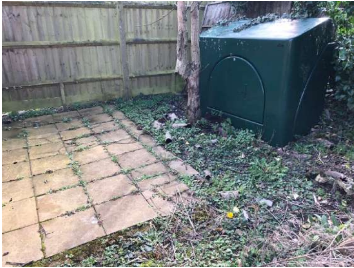
Photo 7: Gas box located within the commercial bin storage area. Note: a broken metal pipe (assumed to be a gas pipe) observed on the right corner.
